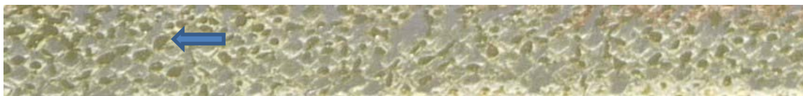
Figure 22. Photograph of a helicopter adhesive bonded joint. Porosity appears as the darker spots throughout the adhesive such as the one indicated by the arrow.
